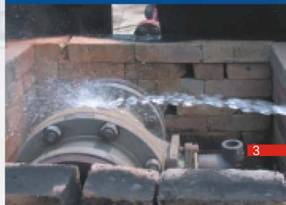
Valve after Test
